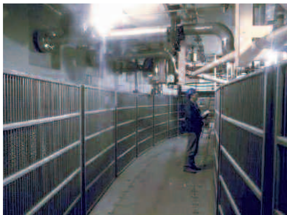
N4 plant series reactor sumps
