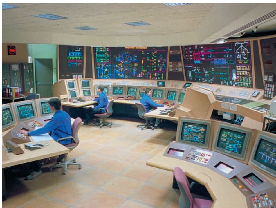
N4 reactor control room
