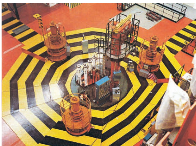
PHÉNIX reactor platform
